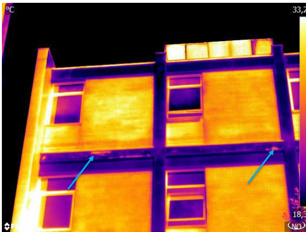
Figure 22 – areas with higher temperature, which identify the detached plaster
